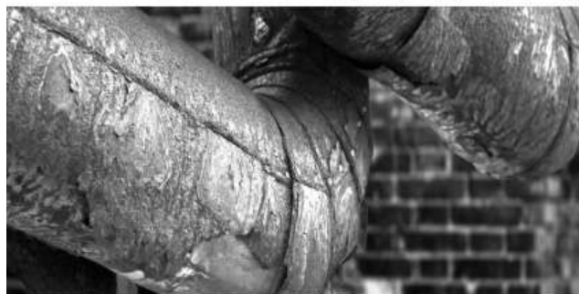
Figure-1. Corrosion affecting the metal structure
