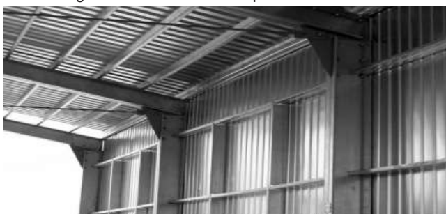
Figure-3. Formation of steel corrosion
